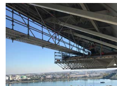
Suspended Access Platforms
