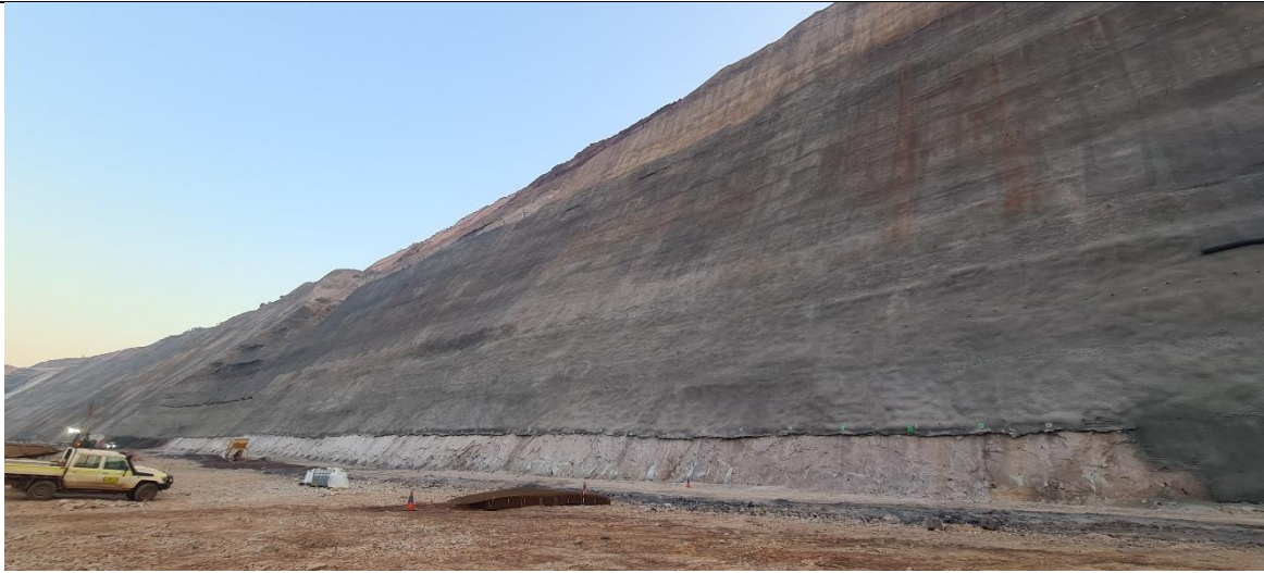
WD8 rigid meshing section. 170x sheets of rigid mesh, shotcrete and cable bolts done over the week.
